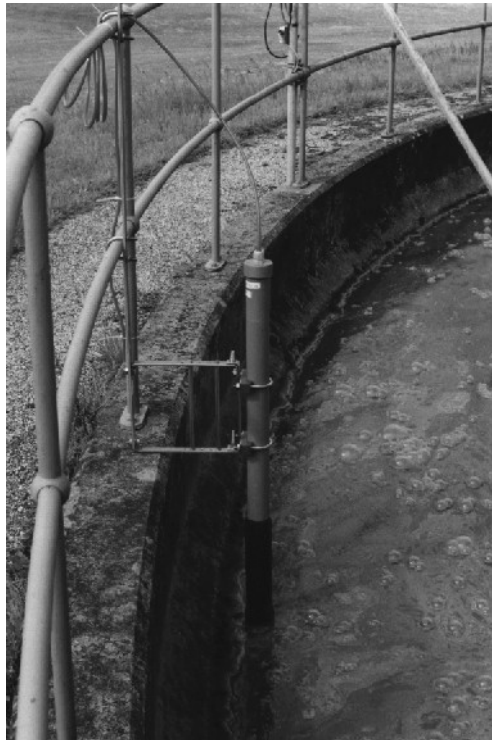
Figure 2 Typical TT2000 Installation
